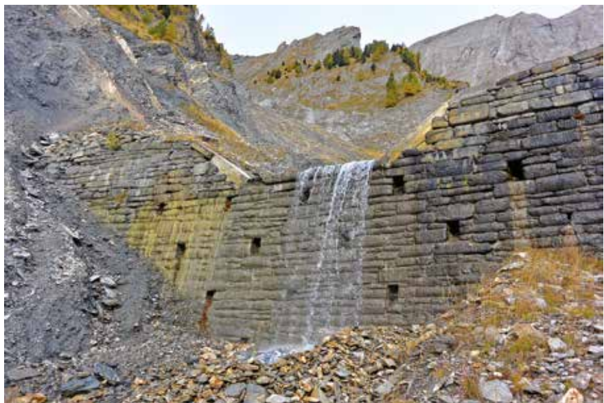
Fig. 6 – Torrential barrier of 23.5 m height.
